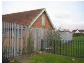
L. High perimeter fencing to Community Centre for security
