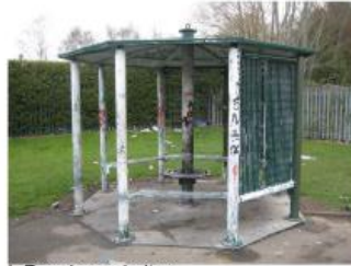
I. Run down shelter
